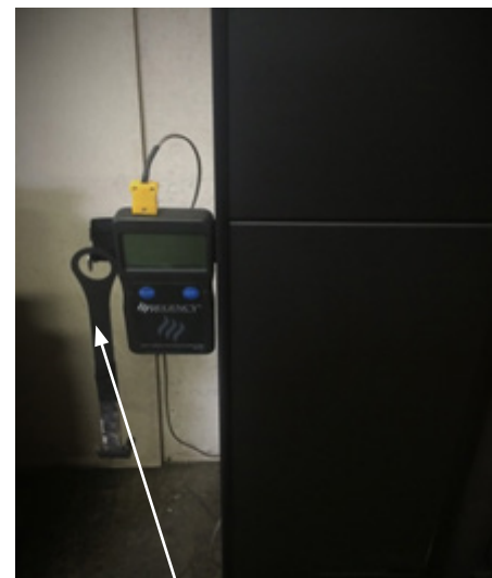
Air and Bypass operating handle/monitor storage.
