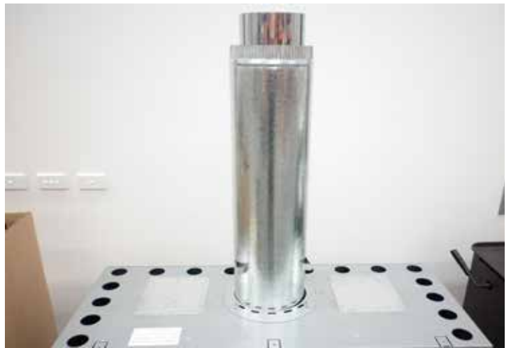
4. 10" galvanized flue skin fitted. The 10" skin sits on top of the box over ventilation holes in plate. Note: Crimped end is up.
